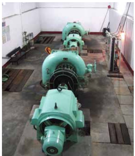
View of the turbine hall of one of the Chongqing based projects.
