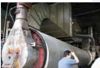
Heavy Oil Burner 2
