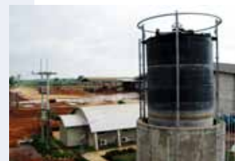
5 Upflow Anaerobic Sludge Blanket (UASB) Biogas Reactor
